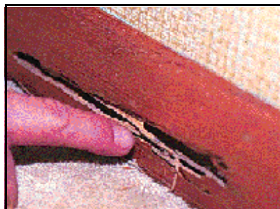
TERMITE DAMAGE TO BASEBOARD. HIDDEN INFESTATION WAS DISCOVERED WHEN VACUUM CLEANER ATTACHMENT PENETRATED SURFACE OF BASEBOARD. (M. Potter, University of Kentucky Entomology)
